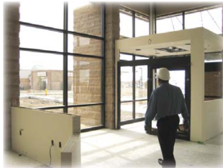
John Reid, MCPN's vice president of development, walks through construction of a new clinic that will double the capacity of MCPN's clinics in Aurora, Adams and Arapahoe counties
